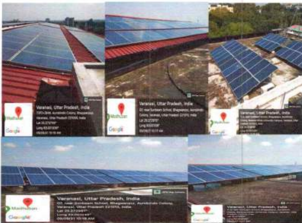
Image 6. Installed Solar panels at college building roof
